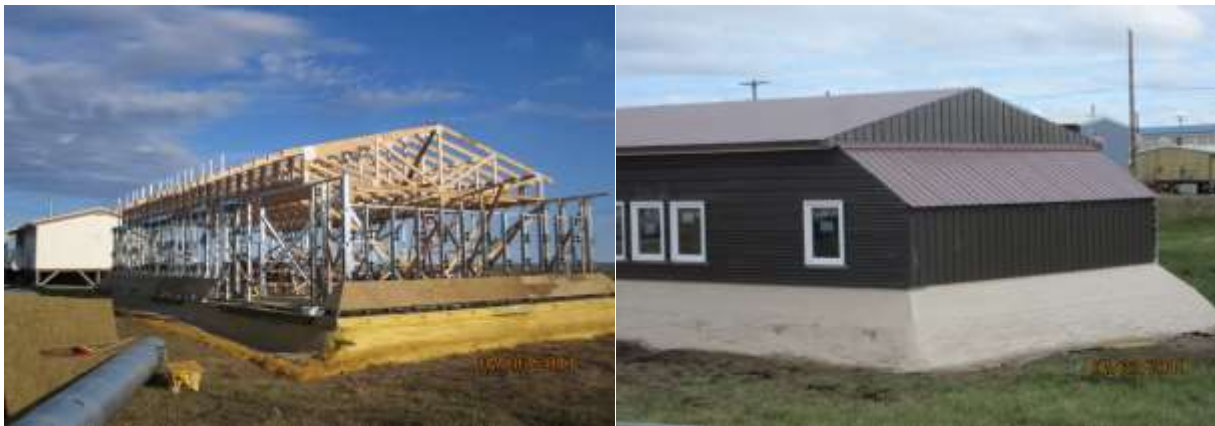
Figures 138 and 139: Under construction and the finished building with the parged raft foundation (CCHRC)
