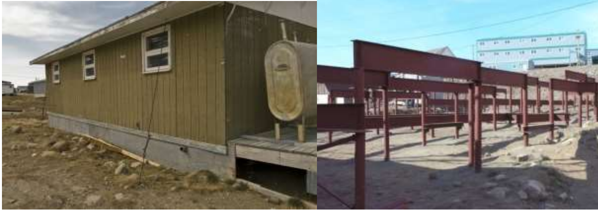
Figure 140 and 141: Cables holding a house to the ground in Nunavut and a pile foundation for a new structure in Iqaluit (Barriault 2011)
