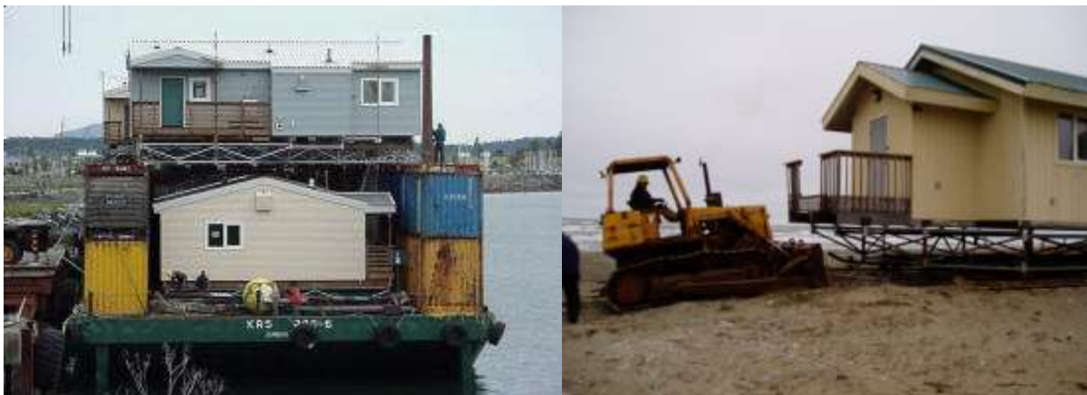
Figures 114 and 115: Barging and pulling houses on tridetic foundations (retrieved from http://multi-point-foundations.com/ )
