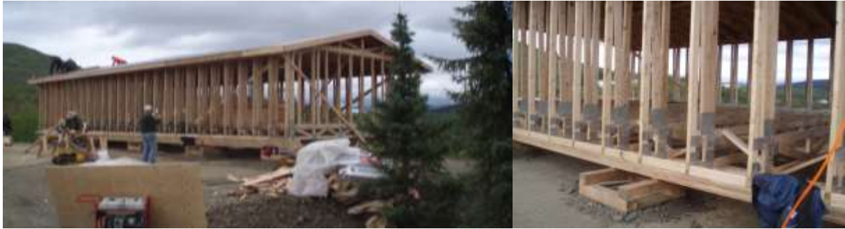
Figures 136 and 137: When finished, the structure allows for a super energy efficient building envelope (Hebert 2012)
