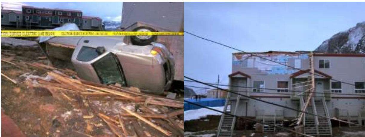
Figures 131 and 132: Wind damage to vehicles and buildings under construction (Nunavut Housing Corp)
