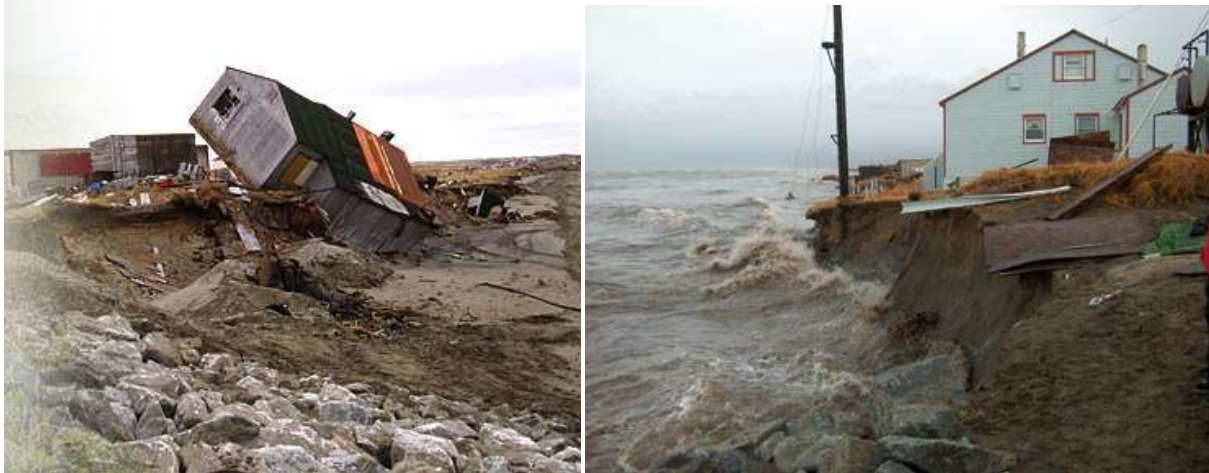
Figures 112 and 113: Impacts of Coastal Erosion in Shishmaref, Alaska (retrieved from http://multi-point-foundations.com/ )
