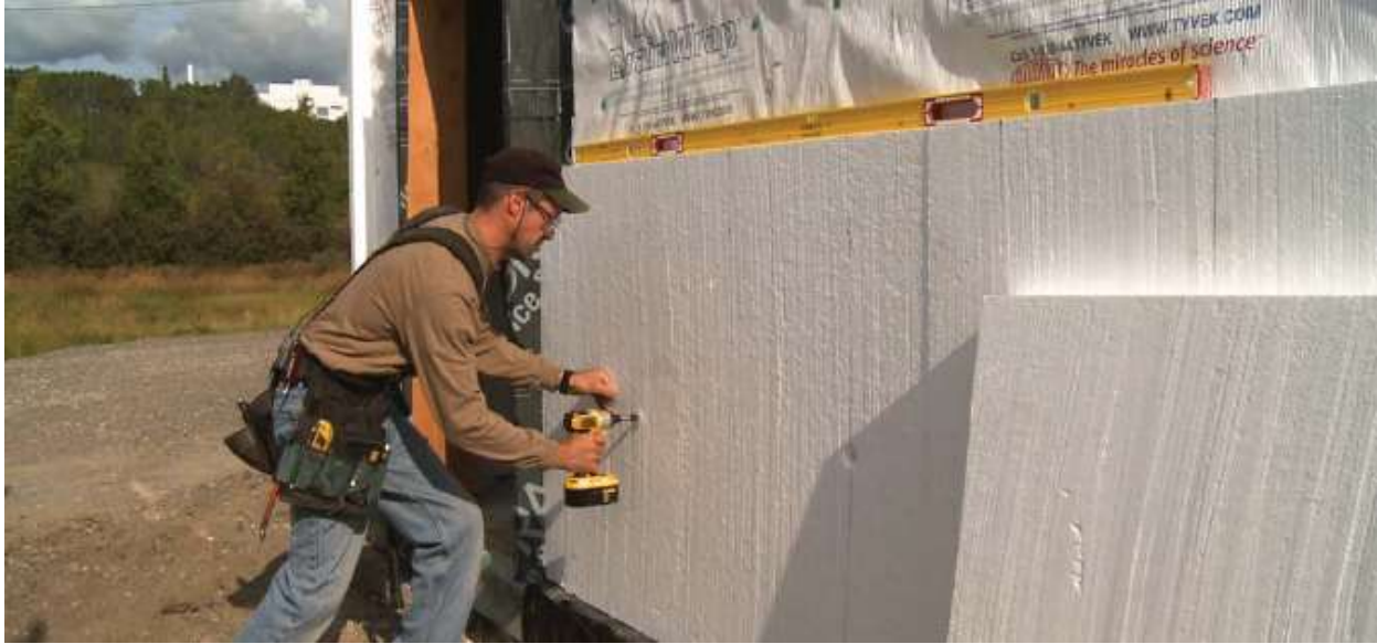
Figure 57: Installation of continuous exterior insulation as part of the REMOTE Wall (CCHRC 2009)
