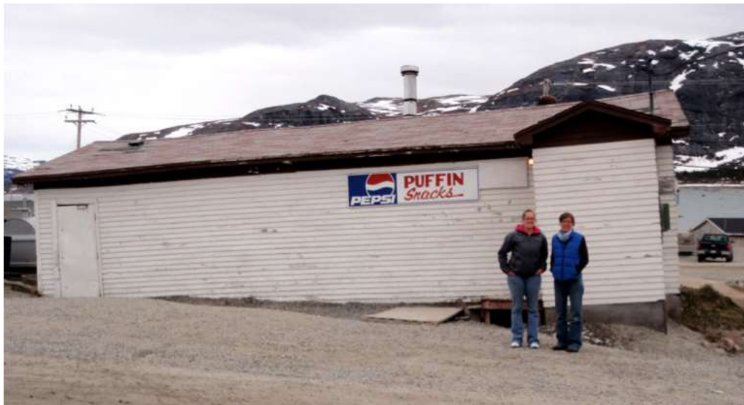
Figure 2: Ground subsidence related to permafrost thaw causing structural damages and infrastructure maintenance issues in Nain, Nunatsiavut. Photo: Trevor Bell
