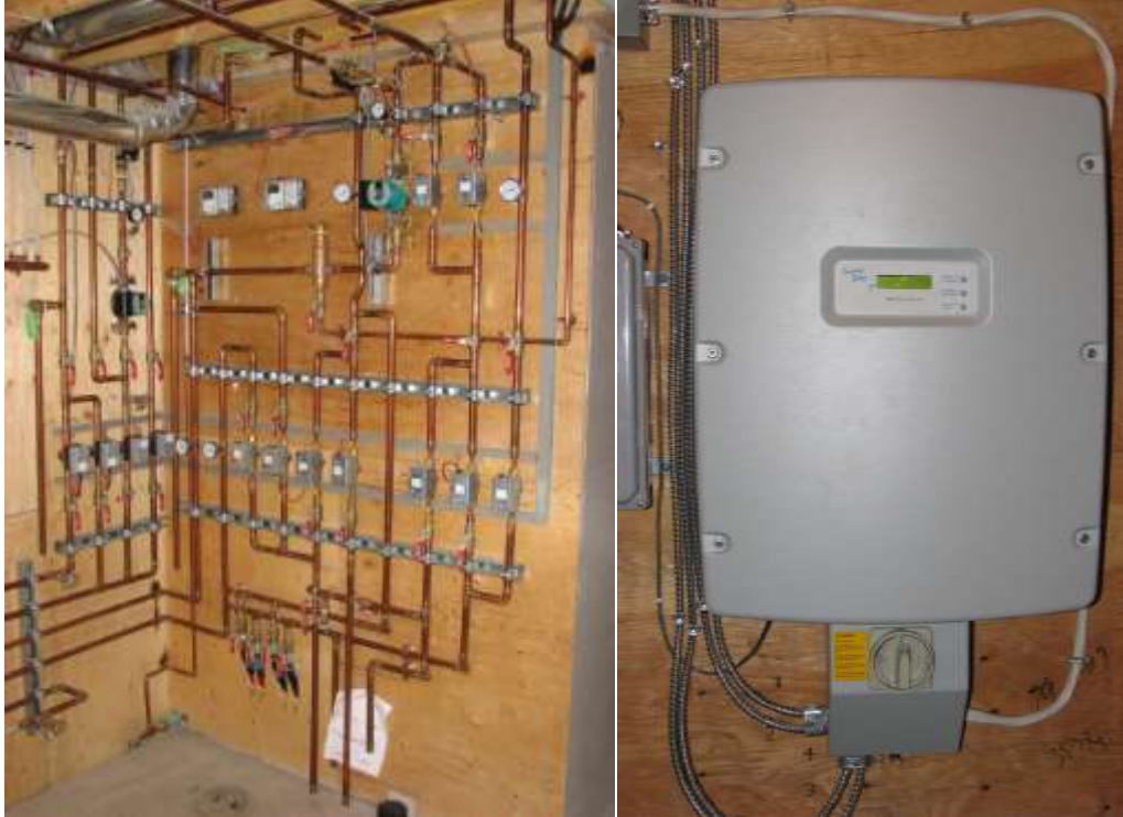
Figures 87 and 88: Riverdale EQ: Piping for the thermal system; and inverter for photovoltaic system (Howell 2010).
