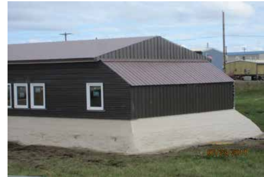
Figure 138 and 139: Under construction and the finished building with the parged raft foundation (CCHRC)
