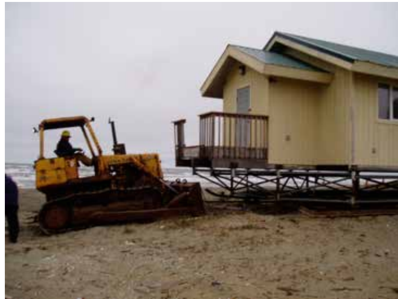
Figures 114 and 115: Barging and pulling houses on tridetic foundations (retrieved from http://multi-point-foundations.com/ )
