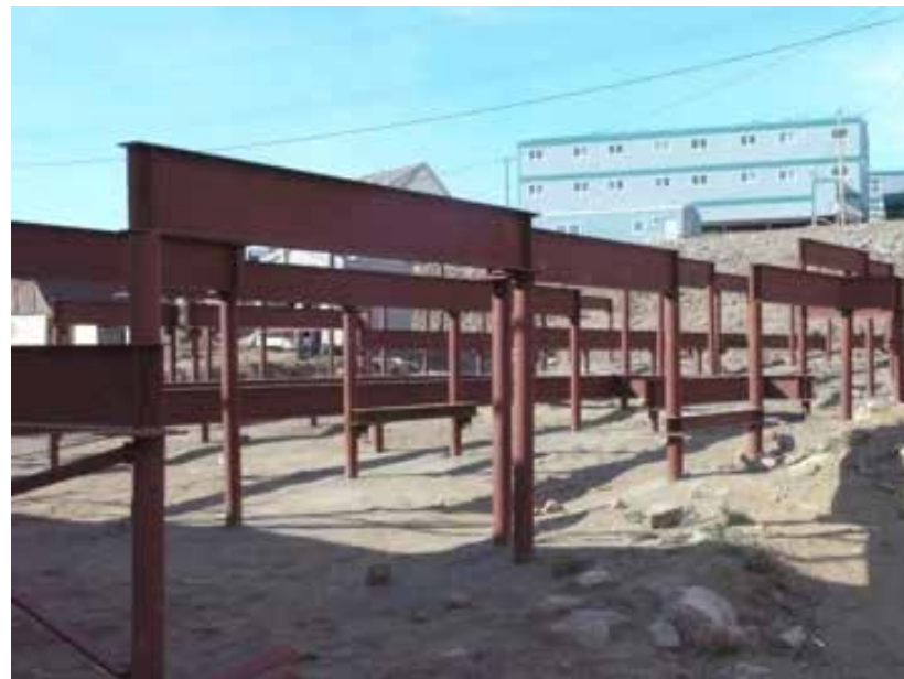
Figure 140 and 141: Cables holding a house to the ground in Nunavut and a pile foundation for a new structure in Iqaluit (Barriault 2011)
