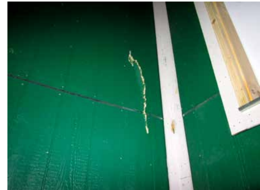
Figures 133 and 134: In the distance two SIP's houses withstand the ravages of the storm with minor damage to the exterior from flying debris (Nunavut Housing Corp)
