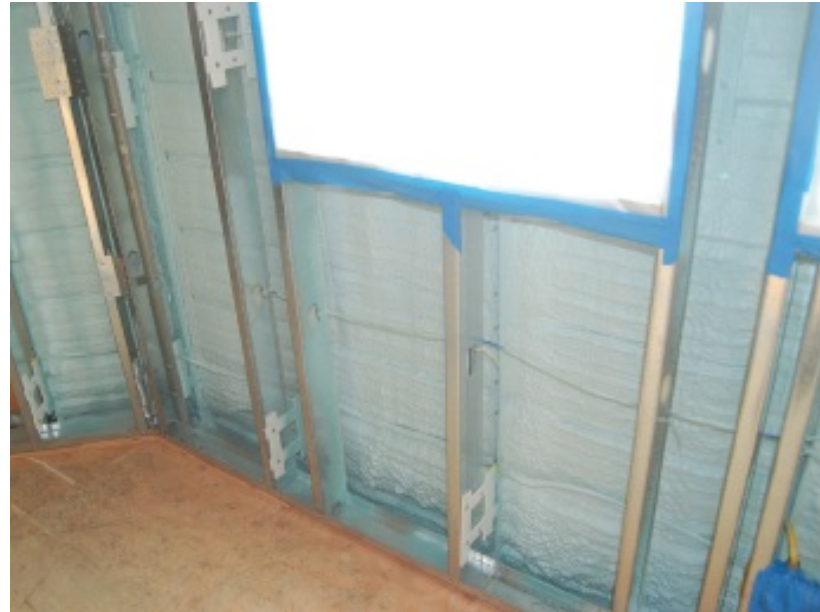
Figures 127 and 128: The rood truss tension bracket and off set wall with bracing (CCHRC 2011)
