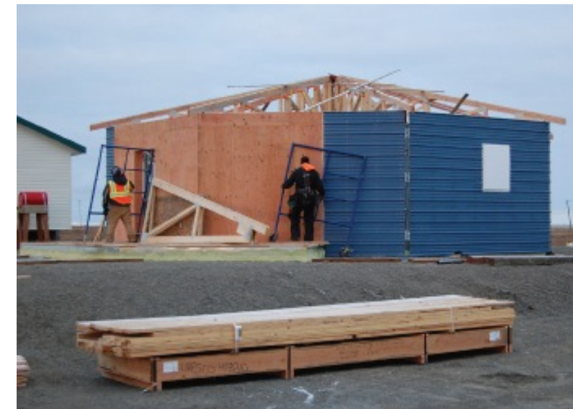
Figures 125 and 126: Location of Quinhagak and the assembling of the Northern Sustainable Shelter Project (CCHRC 2011)
