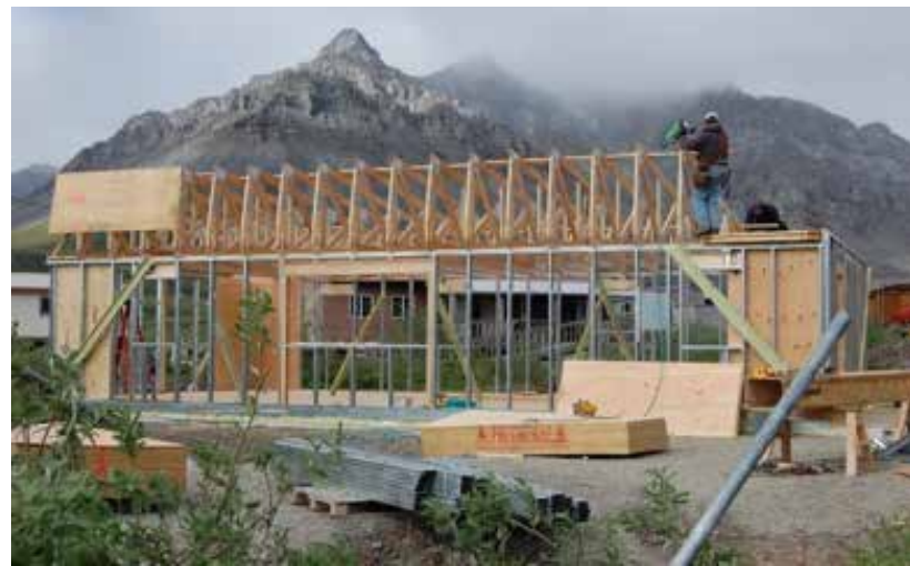
Figures 31: The framing system underway on site, and spray foam insulation being added to the exterior of the house. (Hebert, 2010)
