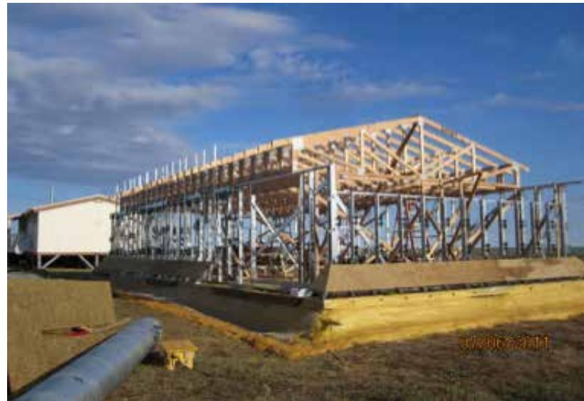
Figure 138 and 139: Under construction and the finished building with the parged raft foundation (CCHRC)
