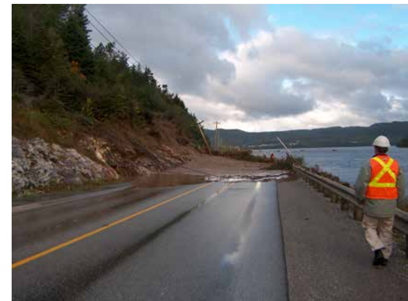
Figure 3-2. Landslides on coast at Southern Harbour 2010. Source: Liverman, D., Batterson, M., and Taylor, D. 2013. Geological Disasters in Newfoundland & Labrador . Retrievable online at www.nr.gov.nl.ca/nr/mines/outreach/geologicalhazard.html , last accessed on April 1st 2013.
