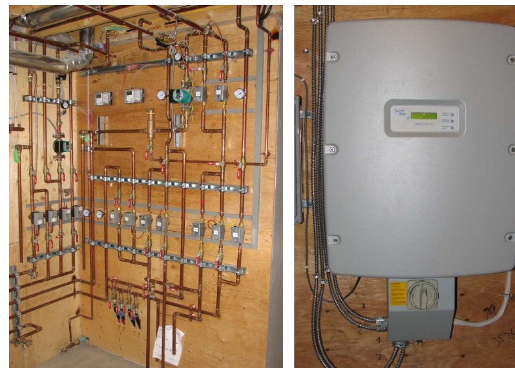
Figures 87 and 88: Riverdale EQ: Piping for the thermal system; and inverter for photovoltaic system (Howell 2010).
