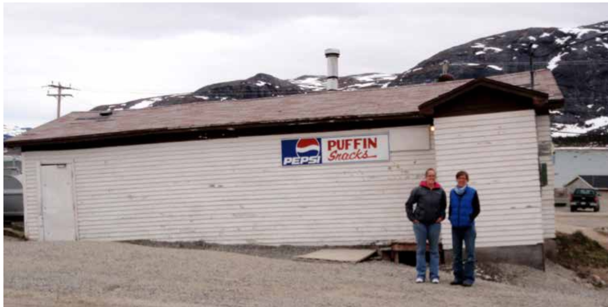
Figure 3-1: Ground subsidence related to permafrost thaw causing structural damages and infrastructure maintenance issues in Nain, Nunatsiavut. Photo: Trevor Bell
