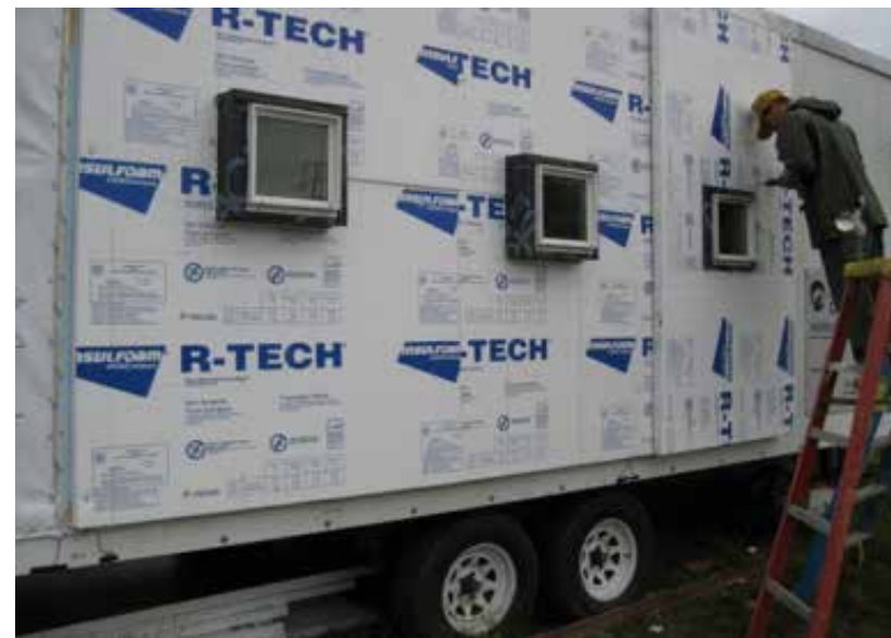
Figures 69 and 70: REMOTE Wall Details and the CCHRC Mobile Test Facility (CCHRC 2010)
