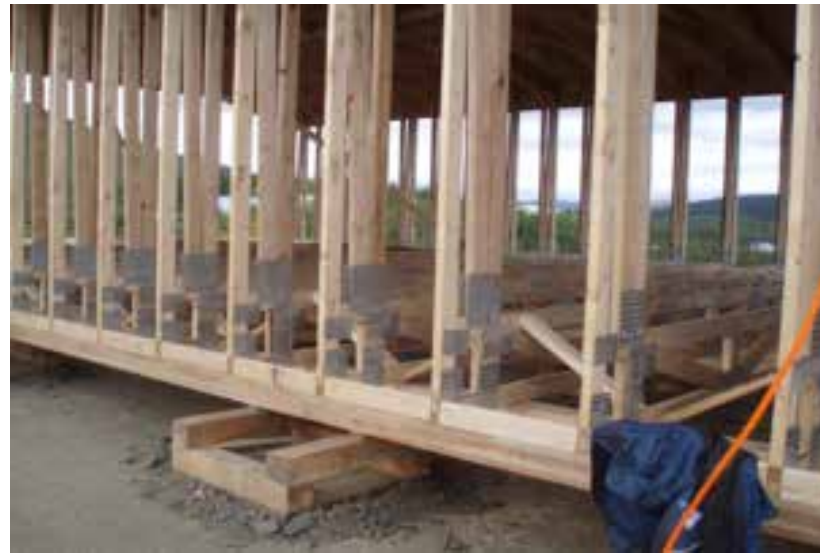
Figure 137: When finished, the structure allows for a super energy efficient building envelope (Hebert 2012)
