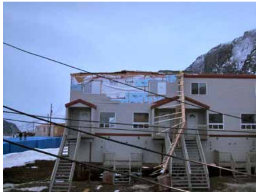
Figures 131 and 132: Wind damage to vehicles and buildings under construction (Nunavut Housing Corp)
