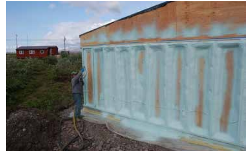
Figures 32: The framing system underway on site, and spray foam insulation being added to the exterior of the house. (Hebert, 2010)
