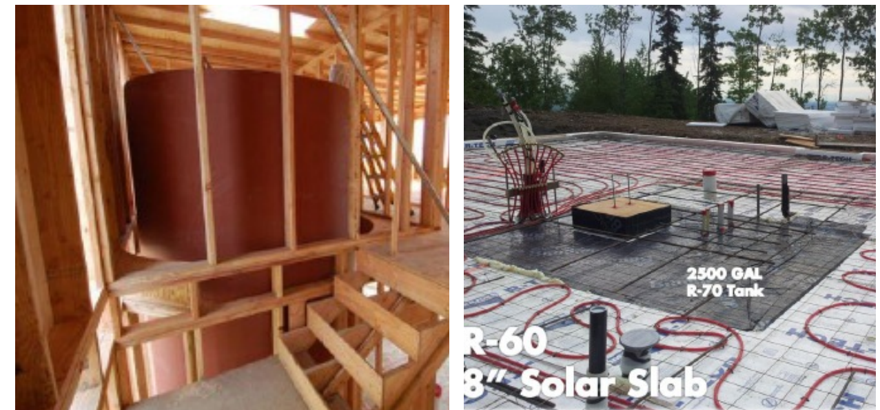
Figures 92 and 93: Residential thermal storage tanks in Fairbanks. Photos courtesy of Reina, LLC.
