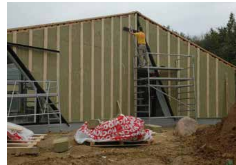
Figures 74 and 75: Wall Retrofit Detail and Exterior Retrofit in Process (Bjarlov & Vladykova 2012)
