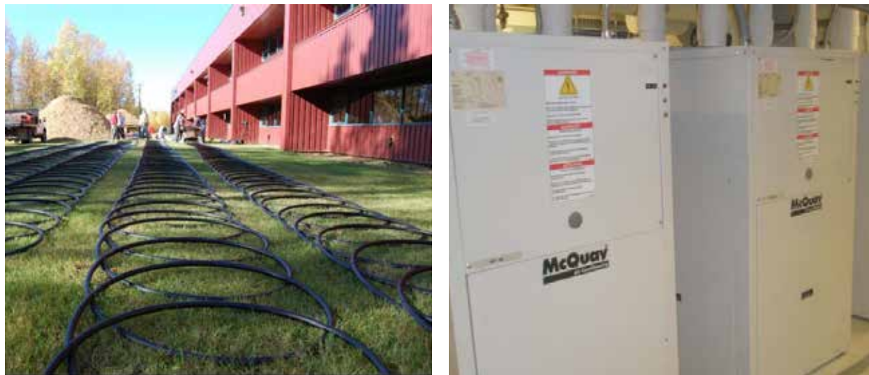
Figures 107 and 108: Ground loops for installation at Weller School and Heat pump units at the Juneau Airport. (Craven et al 2013)
