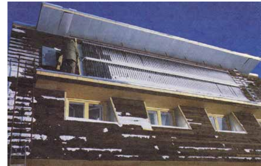
Figure 41: South Elevation - Saskatchewan Conservation House Figure; and Snow Accumulation on the Solar Panels of the Saskatchewan Conservation House (Dumont 2010)
