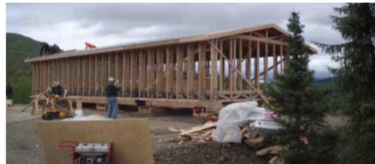
Figure 136: When finished, the structure allows for a super energy efficient building envelope (Hebert 2012)
